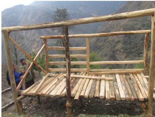
Fig. No. 2.4.3.2 Laying the wooden planks with appropriately so the goat's leg will not pass from holes
