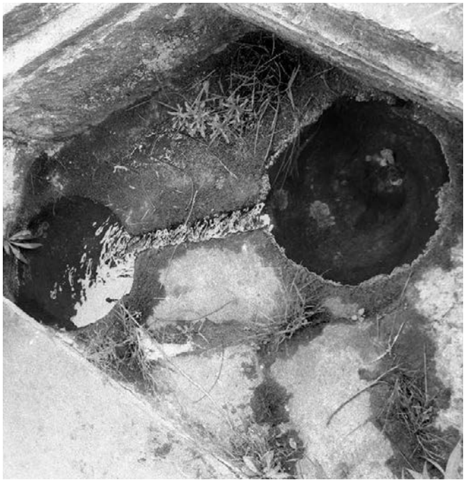
The water comes into the large hole (note the ripples) and runs through the trough into the smaller hole. From there it goes into the building.
