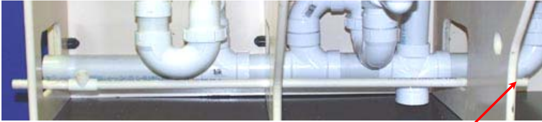
Hot Water Pipe Ends 3 in (8cm) Beyond Hole Predrilled for Shower Hot Water
