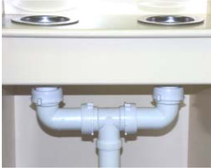
Center Tee Drain Assembly Connected to Basket Strainers
